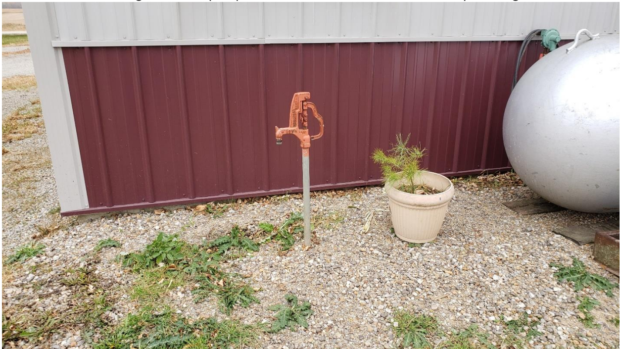
Figure 8 Looking at a water pump behind one of the southern accessory buildings
